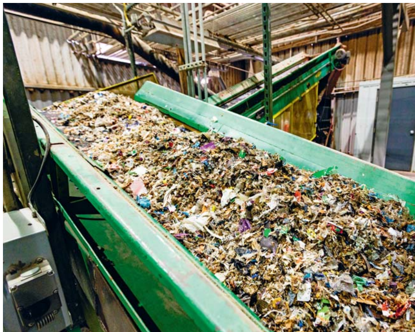
Waste processing unit to produce alternative fuel in our cement plant of Davenport (Iowa, United States)
