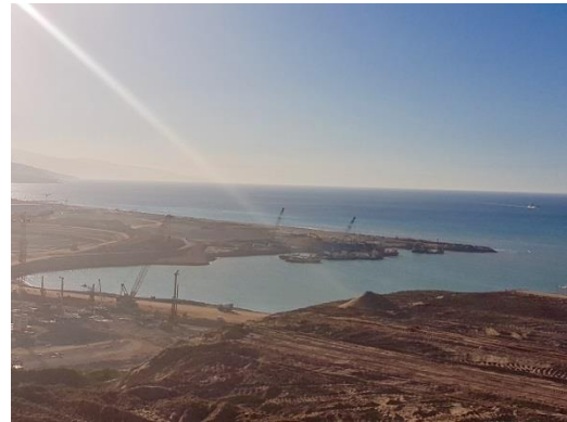
Nador West Med construction site, Morocco Contractor: STFA (Turkey), SGTM (Morocco) and Jan de Nul (Belgium)
